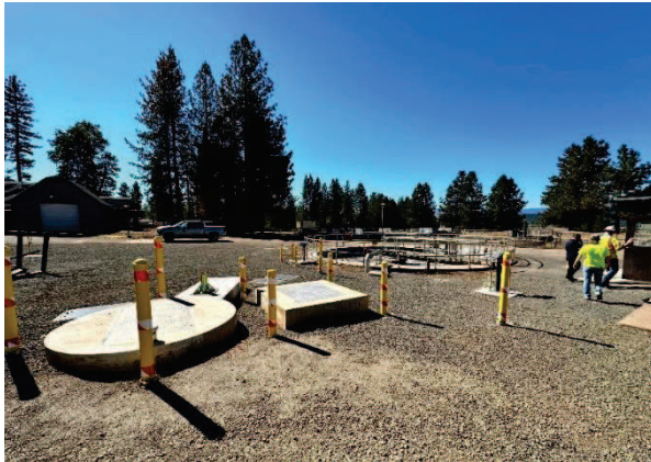
Return Pump Station
