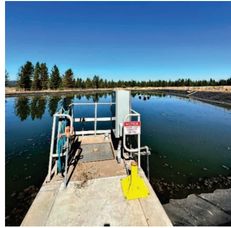
Supernatant Pump Station and Sludge Lagoon
