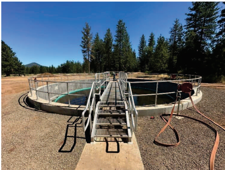
New Secondary Clarifier
