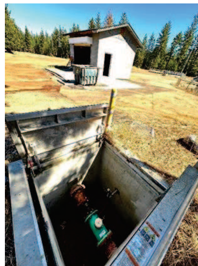
New Flow Meter
