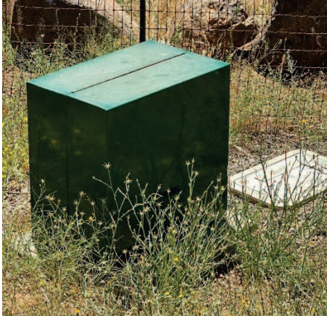
Sludge Lagoon Backflow Preventer and Meter
