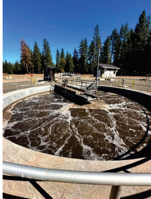
Converted Aerobic Digester
