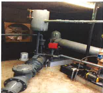
Right-angle drive and vertical turbine pump
